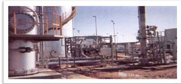
Membrane System for EOR (Enhanced Oil Recovery) installed in Turkey
